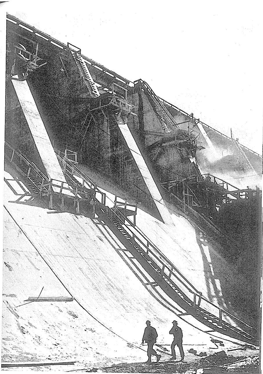
Two construction workers in hard hats walk at the base of the spillways at Fort Loudoun Dam. The curve in the slope is designed so that water passing over the spillways will cause a minimum of erosion in the river channel below.
